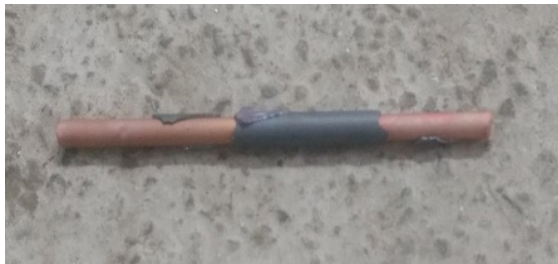
Figure 4. Copper Rod Oxidized
