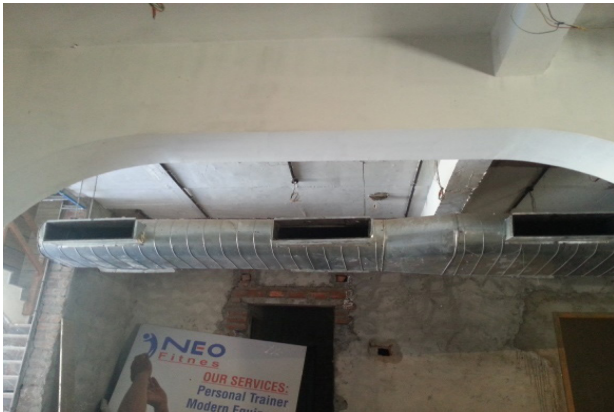
Figure 2. Central air conditioning
