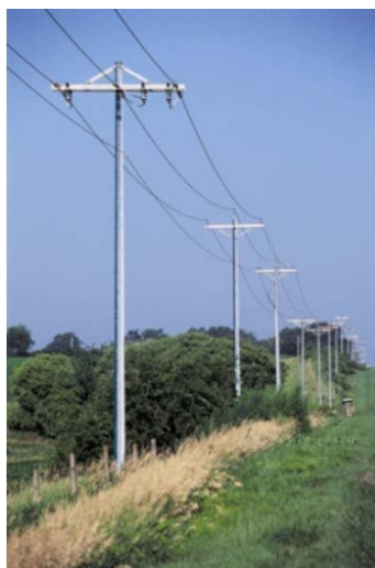
Figure 5. Power transmission line
